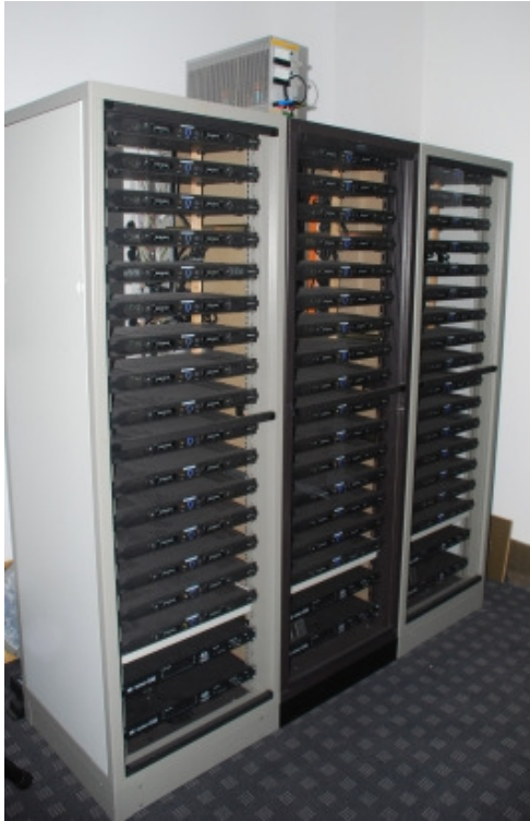
Figure 6: Racks in the control room, containing the DA converters (two units at the bottom of each rack) and the power amplifiers used to drive each loudspeaker of the array with its individual signal.
